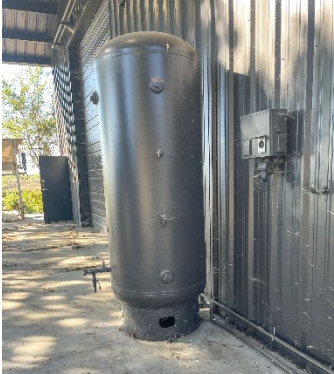
Air Tank/Receiving Tank
